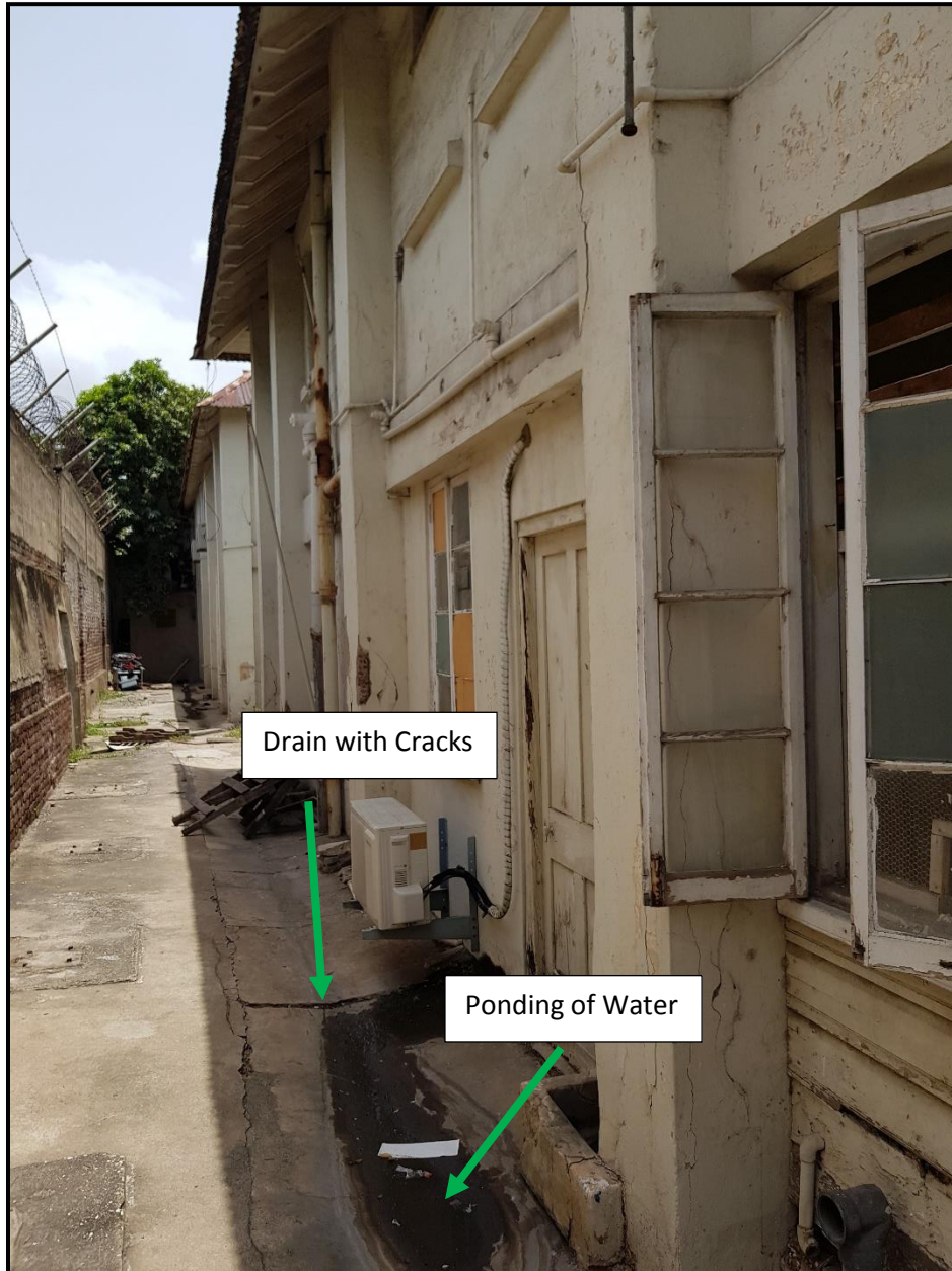
Figure 2. Water seeping into the cracks in the drain.
